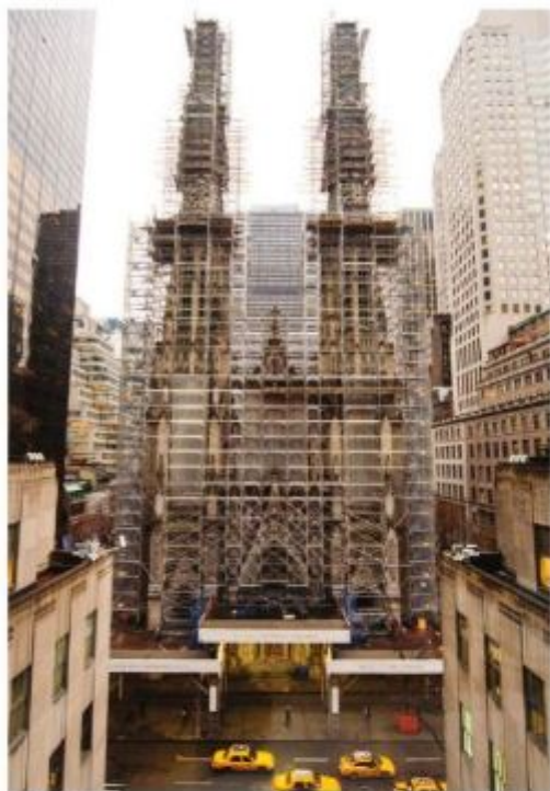
The extensive recent restoration of New York City's landmark St. Patrick's Cathedral, led by Murphy Burnham & Buttrick Architects (MBB), focused on stabilizing the structure and creating a better experience for clergy, visitors, and worshippers. Photo © Chris La Pute
