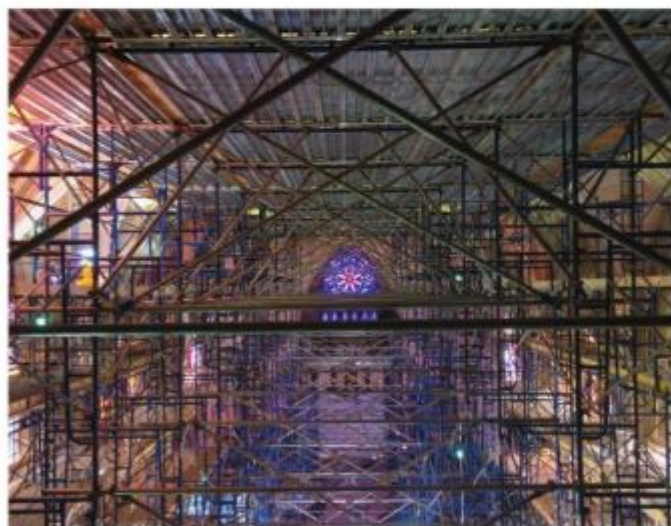
The interface between new interventions and the cathedral's historic elements required a series of carefully considered design decisions about alignments, priorities, and the preservation of the existing architecture, among other factors. Photo © Whitney Cox
