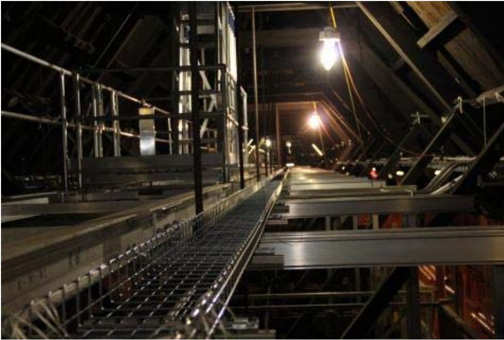
A new fire-suppression system that relies on mist, instead of large amounts of water that would cause structural damage, has been installed.
