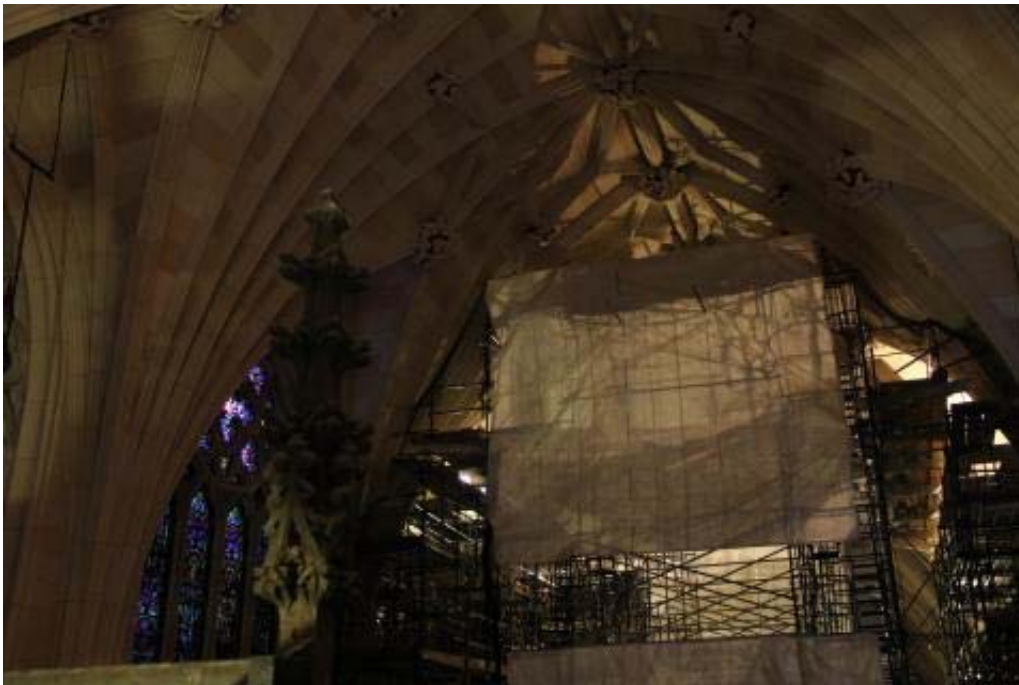
Scaffolding covers the organ loft at the west end of the nave. A number of organ pipes were removed to be repaired, and those that remained were covered to protect them from dust.
